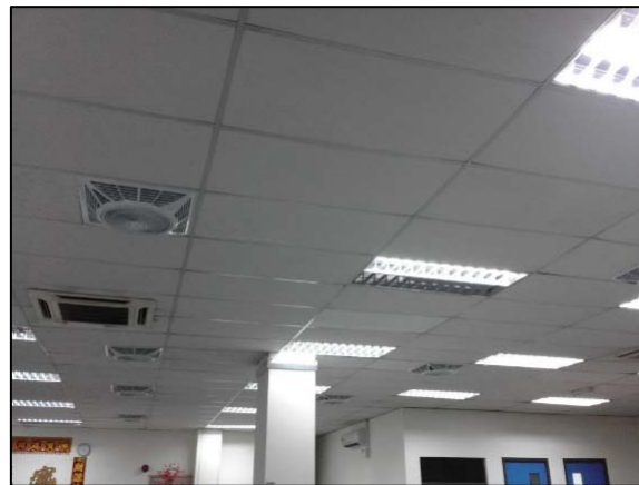
Figure 5: Photo of ceiling fan and direct expansion cassette unit
